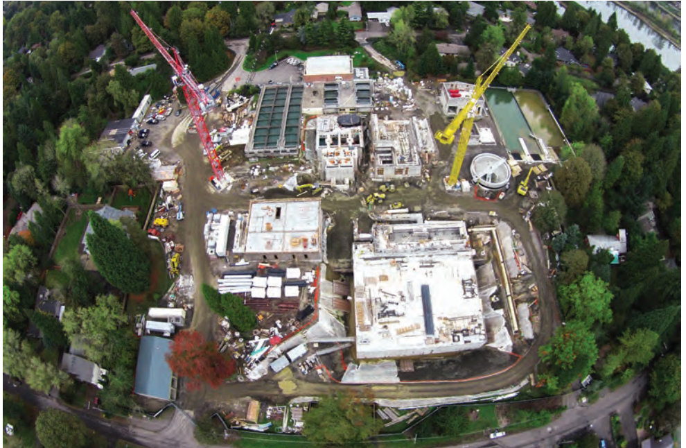
A recent aerial shot shows the water treatment plant that will serve the Lake Oswego-Tigard Water Partnership.
